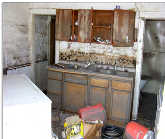
Figure 5-1. A Cedar Rapids home damaged by the 2008 flood. Residents returning to muck out and gut their homes after such events are faced with extensive mold growth, chemical and microbial pollutants, and other potential health hazards. With current rises in precipitation and streamflow, floodplain residents may be increasingly exposed to such hazards. (Photo credit: Linn County Public Health Dept.)
